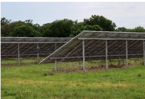
Example of a Solar Conversion System, Ground-mounted
