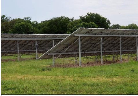
Example of a Solar Conversion System, Ground-mounted
